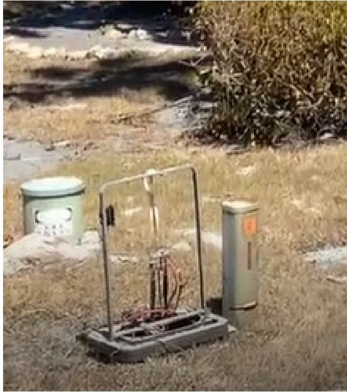
Figure 11 – Pedestal Node Location – Post-Hurricane
