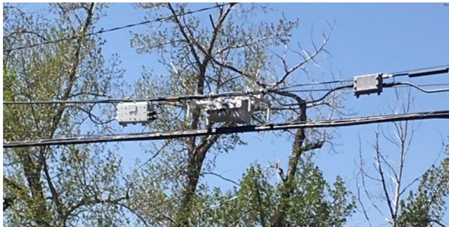
Figure 11 - Small Cell with Demarcation Gateway (Author's Photo)
