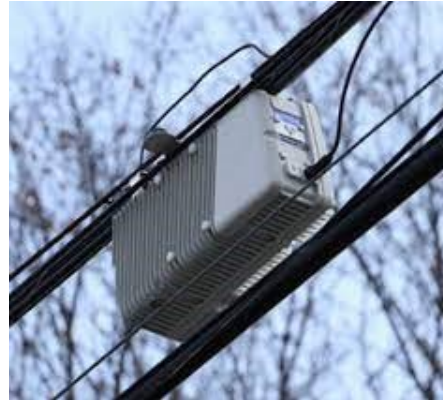
Figure 5 - Small Cell Radio within Communications Space 20
