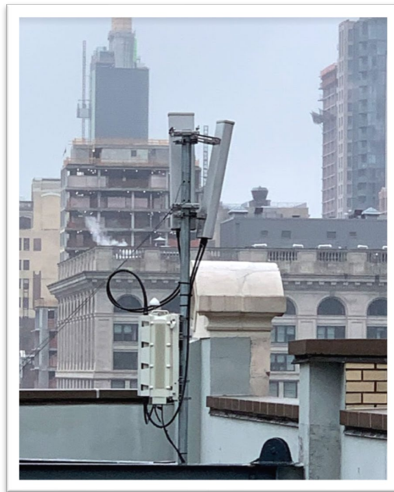
Figure 4 Attached Mount (Rooftop) Outdoor Deployment
