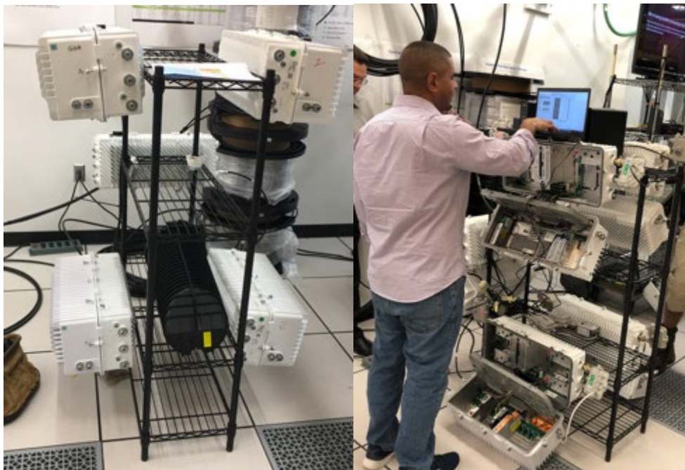
Figure 7 – GOA and GOTs assembled in the headend, Closed (Left) - Open (right)
