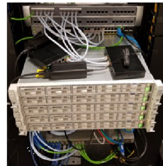
All mounted units shown are connected via Cat6 Ethernet cable to IDC room where MEC system is installed
