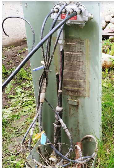
Figure 14 – 412 Test Plant Pedestal
