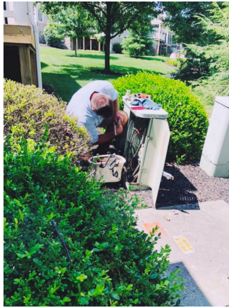
Figure 28. Technician troubleshooting RxMER per subcarrier amplitude ripple.
