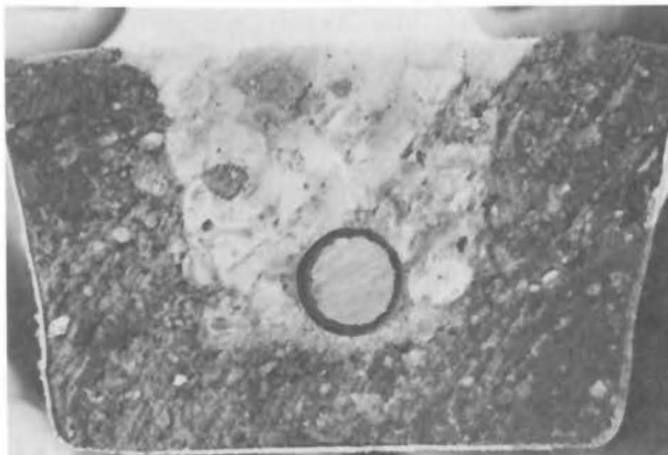
Fig. 20 - Cross-section of PERCOL-encapsulated cable in asphalt pavement, showing intimate bonding of the materials.
