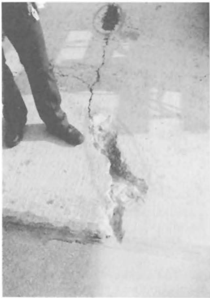
Fig. 6 - Fractured concrete pot-hole on aircraft runway which has been jack-hammered back to solid concrete.
