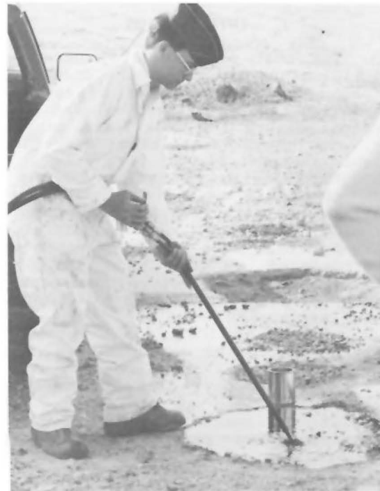
Fig. 2 - Air Force technician floods a debris-filled bomb crater with reactive PERCOL mixture, which gels in two minutes and cures in 30 minutes.
