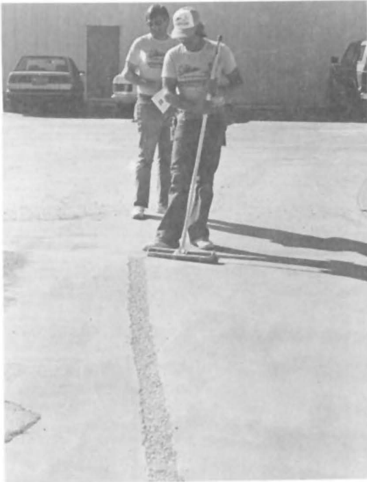
Fig. 16 - Asphalt pavement debris from saw cut is swept back into trench, supplemented by washed, dry pea gravel, cold mix, or recycled asphalt.
