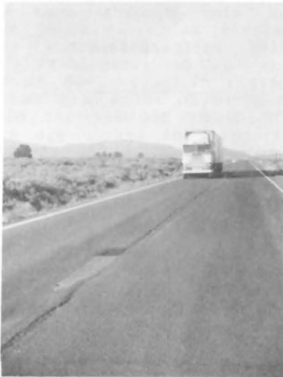
Fig. 3 - Crater (near center line) on U.S. 97 repaired with PERCOL and rock aggregate by California Department of Transportation.
