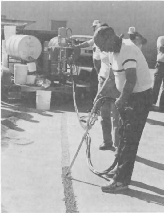
Fig. 18 - Reactive PERCOL mixture flows out of nozzle into trench, percolating through the aggregate and encapsulating the cable.
