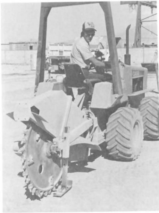
Fig. 14 - 36-inch carbide-tipped Case rock saw used to create 2 3/4 X 6 inch trench in pavement.
