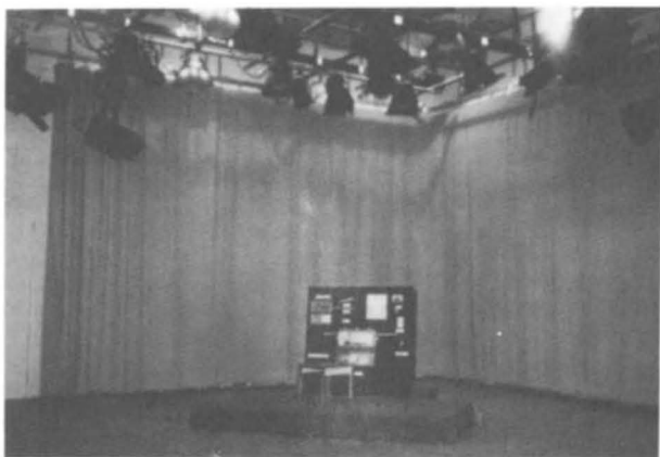
FIGURE 5: TYPICAL LARGE CABLE TELEVISION STUDIO USING CARPET ON THE SPEAKER'S PLATFORM AND HEAVY, FREE-HANGING DRAPES TO REDUCE THE REVERBERATION TIME.
