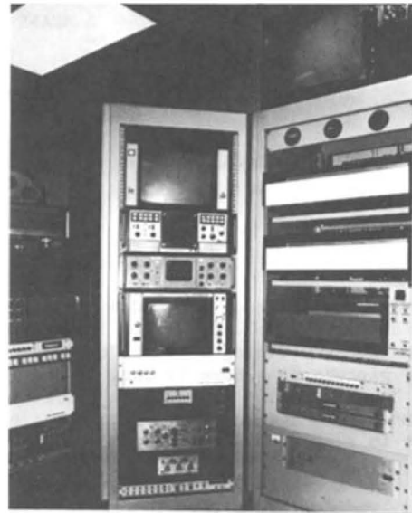
Fig. 7. Recording control and monitoring in center, camera control at left. At right, two of twelve recorders and quality-control player.
